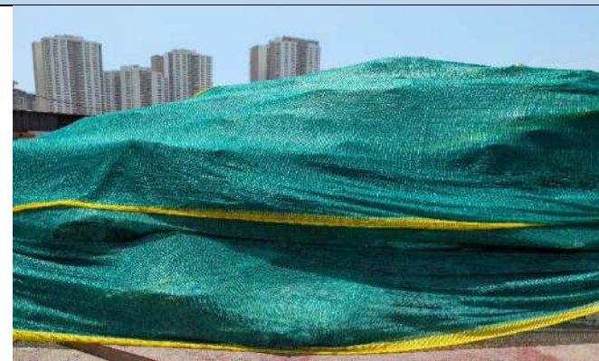
COVERED CONSTRUCTION MATERIALS
